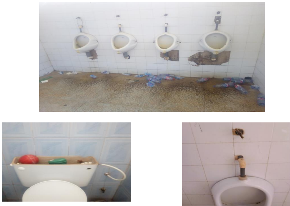
Figure 7: Pictures showing a lavatory in a poor condition, WC cistern with broken flush handle and a stop valve to a urinal (Source: Physical observation)
